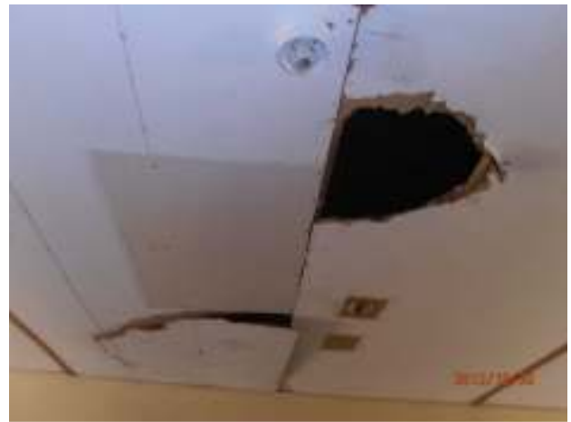
Figure 17 illustrates no bulb and no supply of electricity in the dormitory
