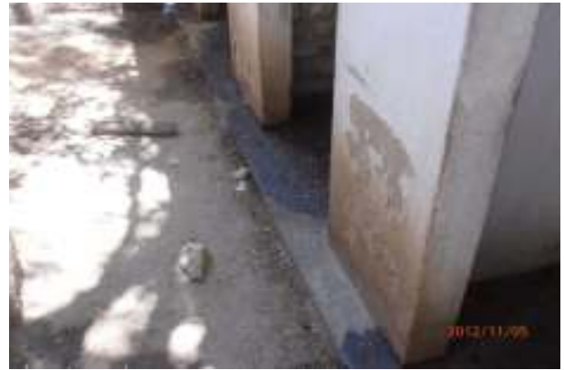
Figure 9 illustrates outside view of the pit latrine condition for San
