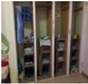
Figure 1 illustrates broken lockers
