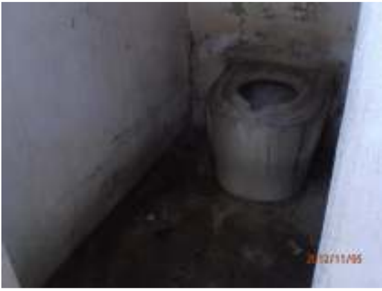
Figure 8 illustrates pit latrine for San
