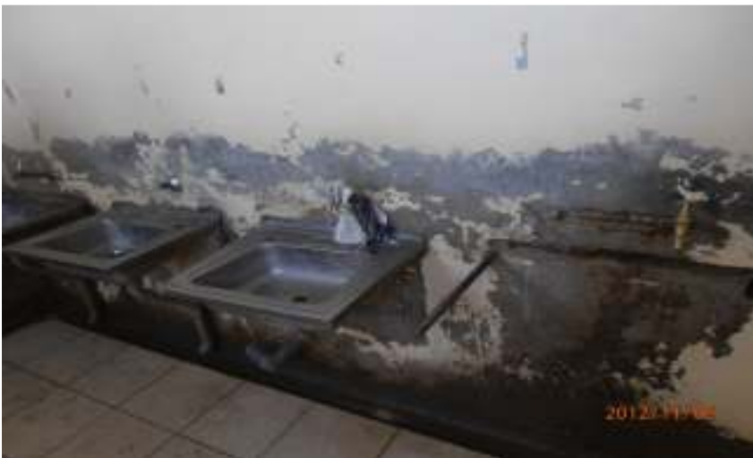
Figure 11 illustrates broken basins and taps
