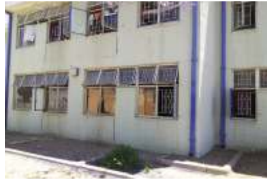
Figure 2 illustrates broken windows
