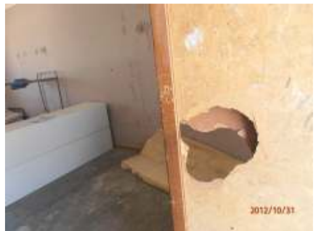
Figure 19 illustrates vandalized door at dormitory
