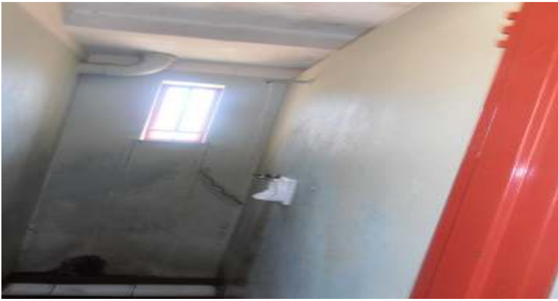
Figure 12 illustrates a broken shower tab with leaking water throughout
