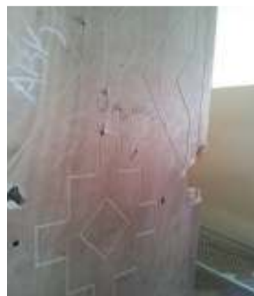
Figure 4 illustrates a broken door
