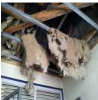
Figure 3 illustrates the condition of the hostels
