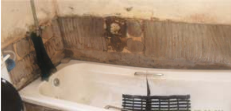
Figure 3: A broken bath tub inside a government quarter in Grootfontein
