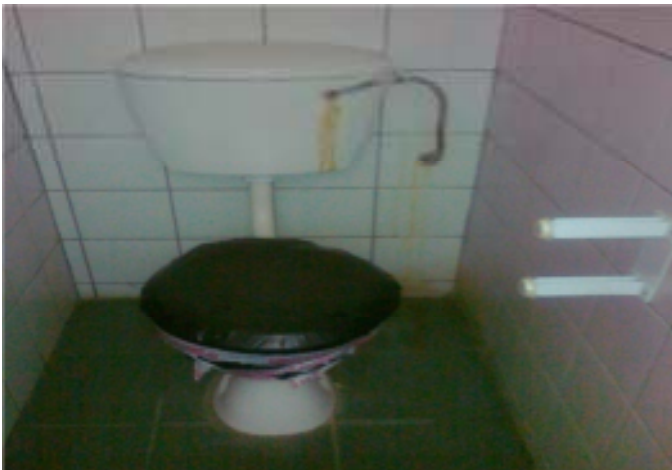
Figure 5: A broken/blocked toilet inside a government quarter in Grootfontein
