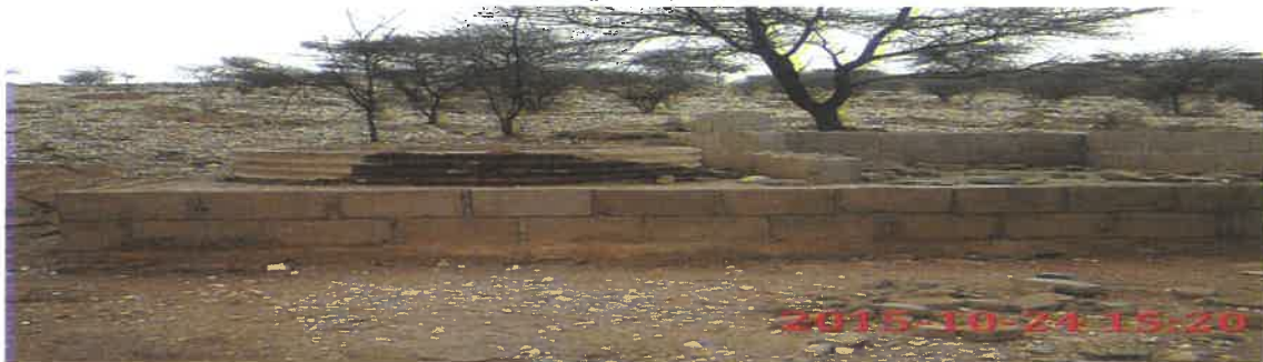
Picture 10: Building not demolished completely
