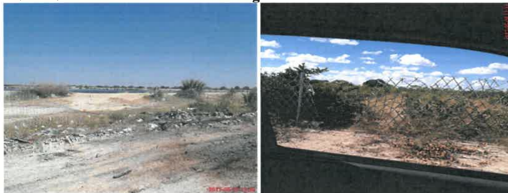
Picture 8: Vandalized Fence at Ondangwa and Rundu
