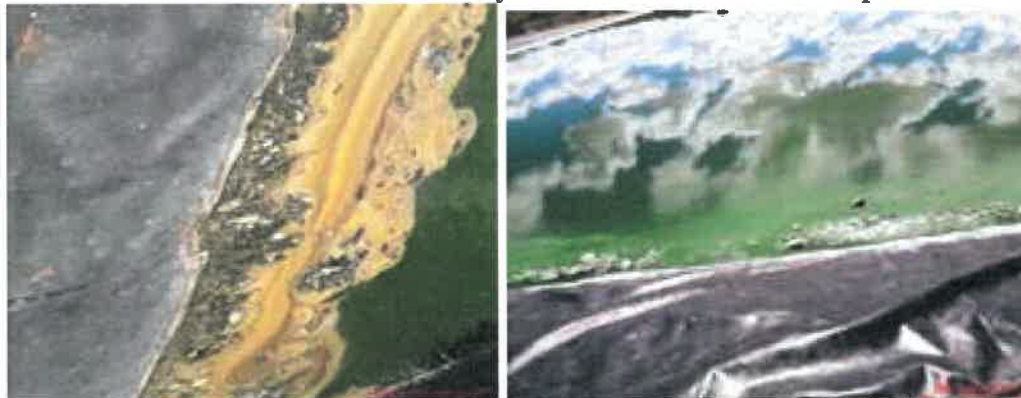
Picture 12: Debris inside the Ponds Systems at Gibeon and Stampriet
