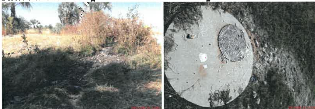
Picture 6: Overflowing Sewer Manholes at Ondangwa and Divundu
