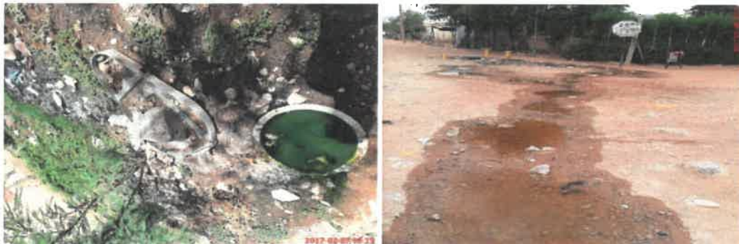
Picture 5: Collection Chambers overflowing into the streets of Gibeon and Stampriet
