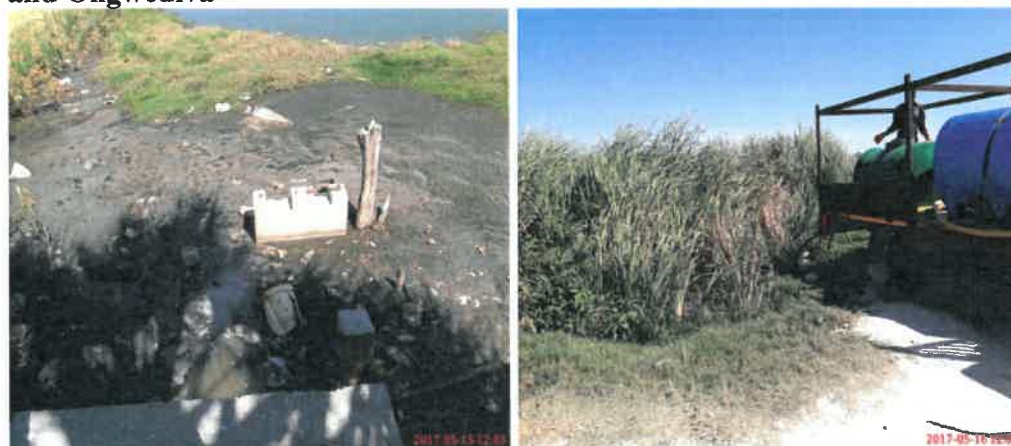
Picture 2: Untreated sewage was disposed-off in unlined Oxidation Ponds at Ondangwa and Ongwediva
