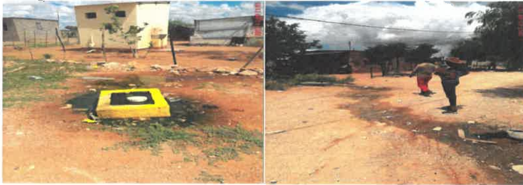
Picture 7: Overflowing Plastic Septic Tanks and Collection Chambers at Kalkrand and Stampriet
