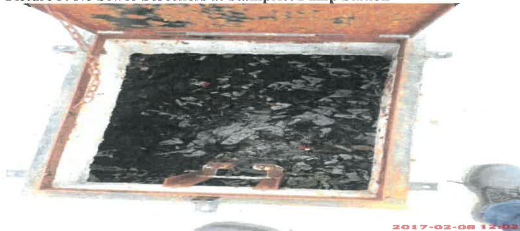
Picture 3: No Sewer Screeners at Stampriet Pump Station
