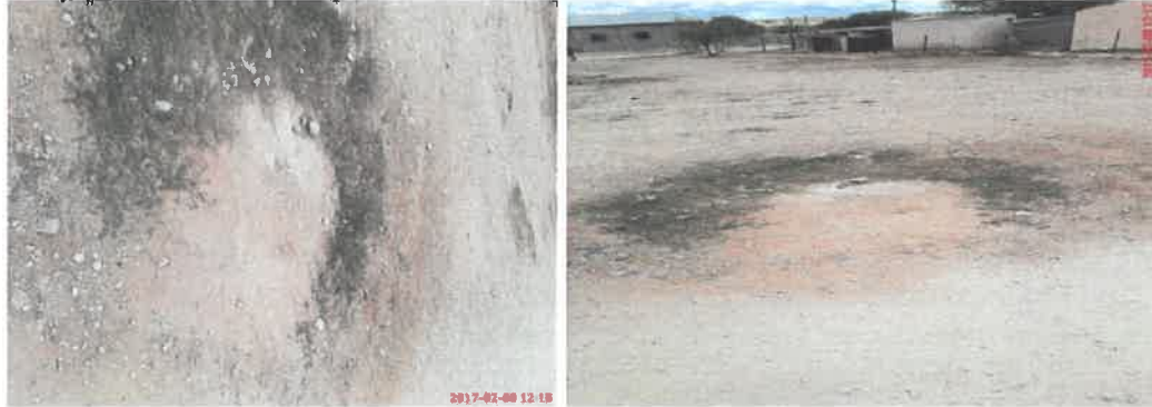
Picture 4: Sewer Manholes in low-lying areas at Stampriet
