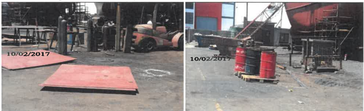
Picture 4: Oil spills and lack of drip trays for oil drums at NAMPORT
